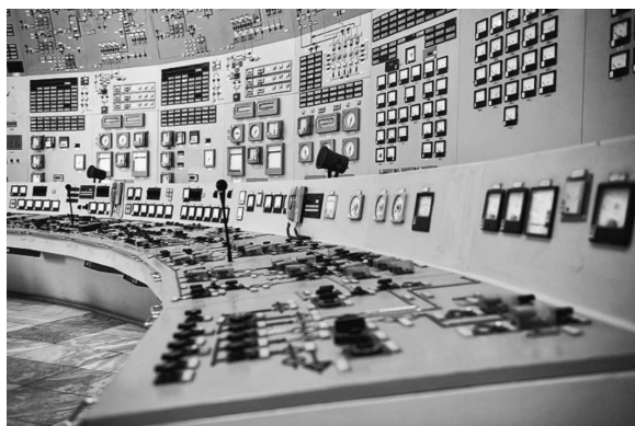
(a) Power plant control room
